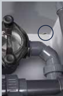
Leaking operating fluids can be drained via the drain cock.
